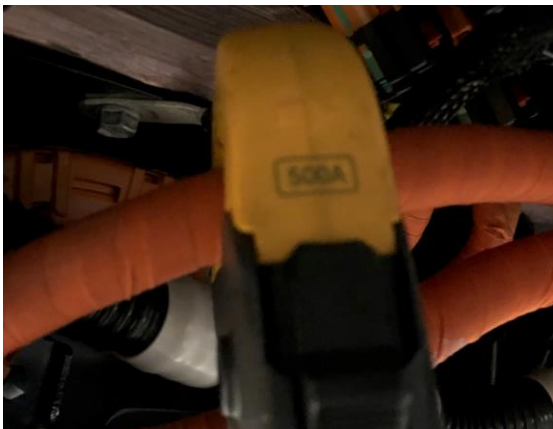
Pic of Hioki connection - Front Motor
