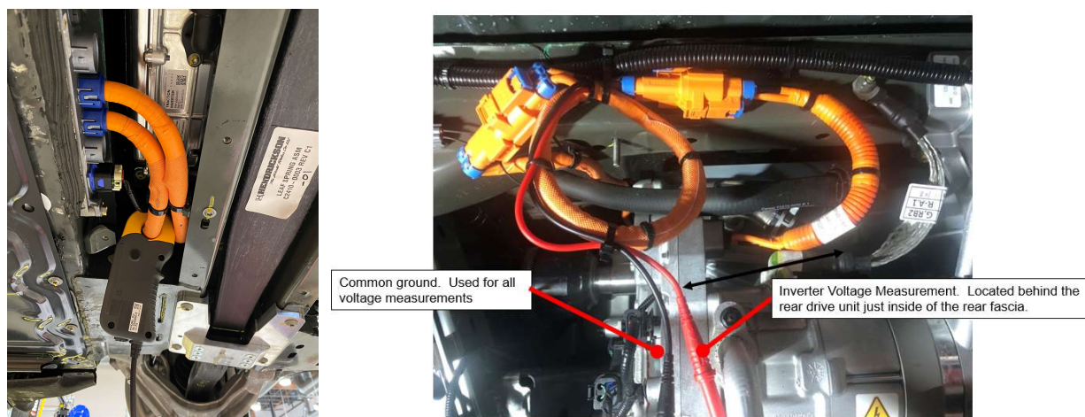
Inverter Current/Voltage Measurement (Rear Drive Unit)
